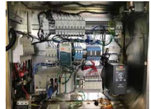
Control Panel Detail
